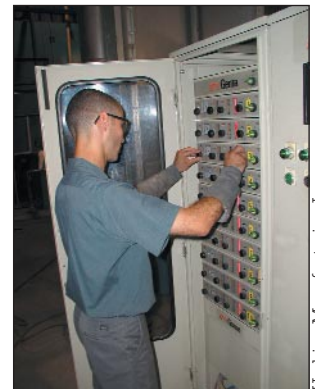
An ITW Gema gun control unit ensures consistent film thickness.
