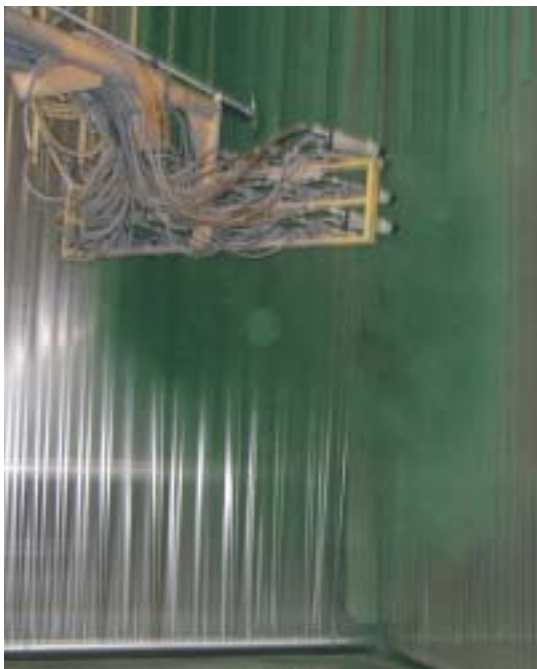
Spray booth walls are changed by indexing a new sheet of plastic.
