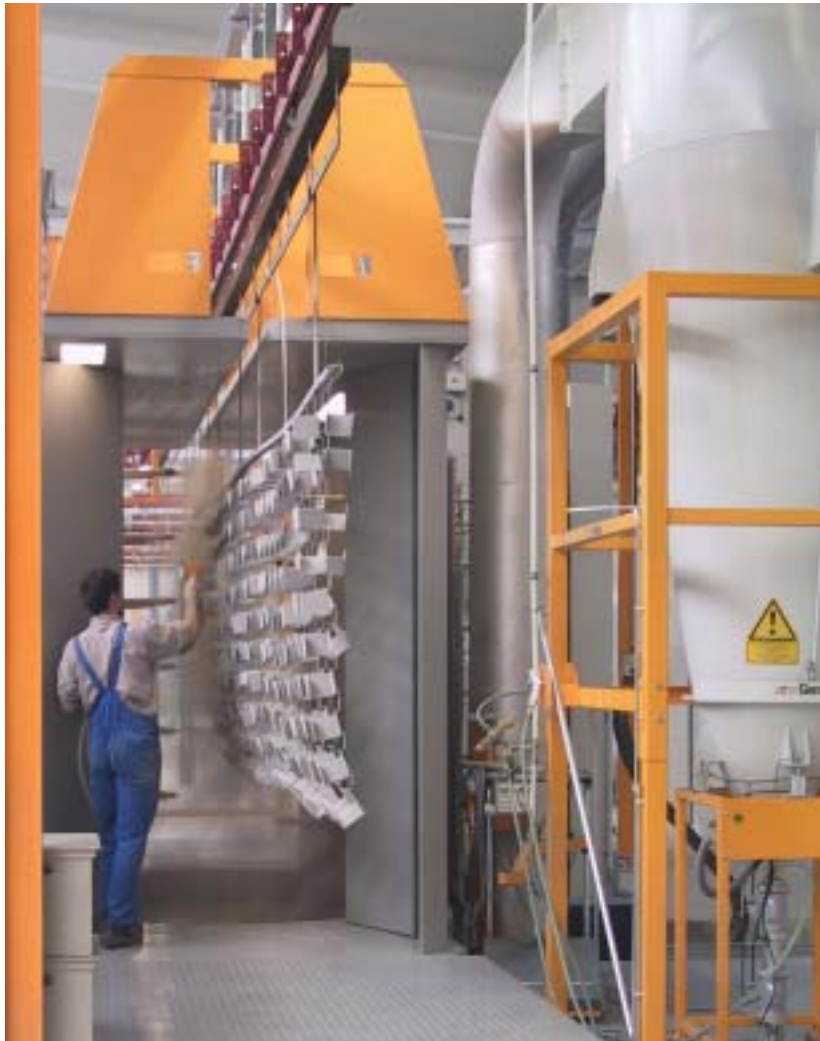
The subcontract coating company Punitec built a new powder coating plant on a 'green field' site, which meant that no compromises had to be made with regard to space planning.
