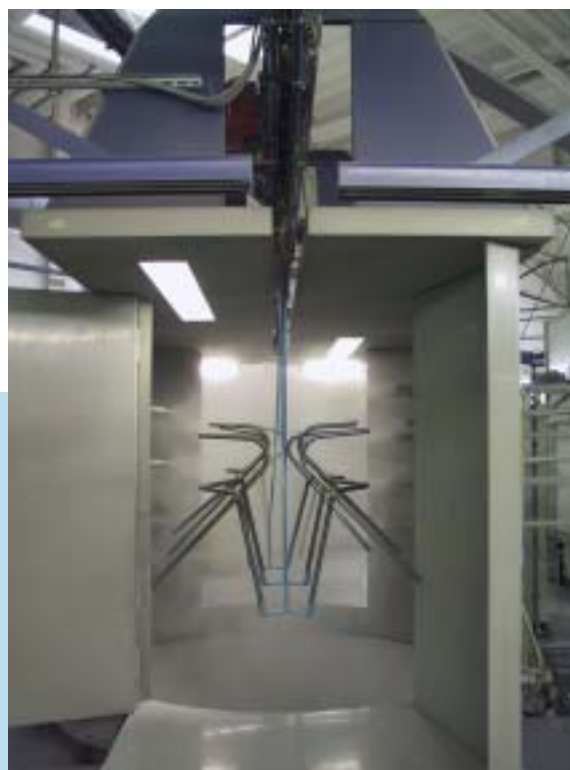
The coating booths were also arranged at an angle at the special furniture manufacturers VS in order to make optimum use of the space available. The unit has a conveying speed of six metres per minute.
