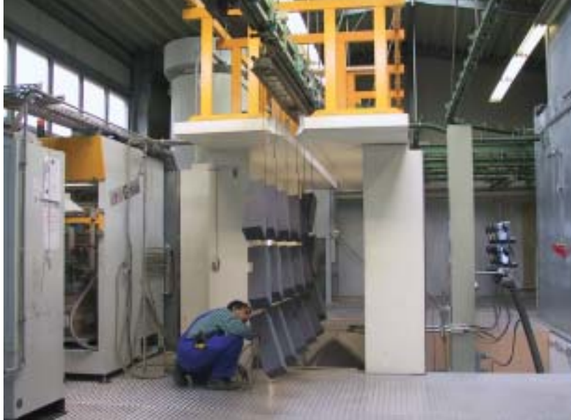
Due to the limited space available, the round cylinder in this application example was transformed into a square booth.
