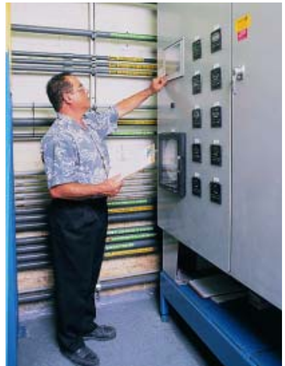
The eco-friendly waste treatment process, controlled by a Quantum PLC, is initiated automatically or manually from the Graphic Magelis operator interface.
