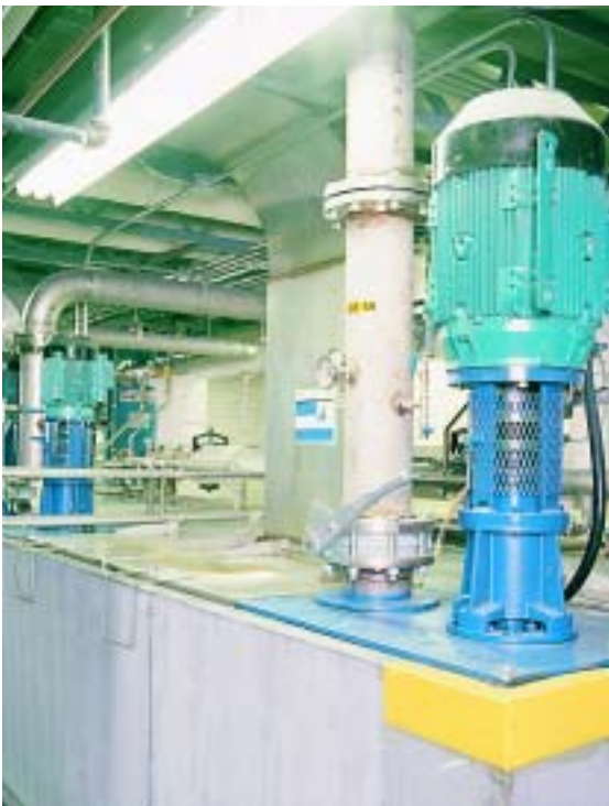
The pretreatment tanks and pumps, located under the mezzanine, supply chemical solutions to the wash.
