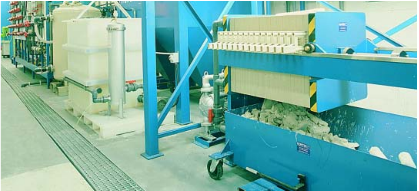
Pretreatment process waste is chemically treated and produces a filter cake for disposal.
