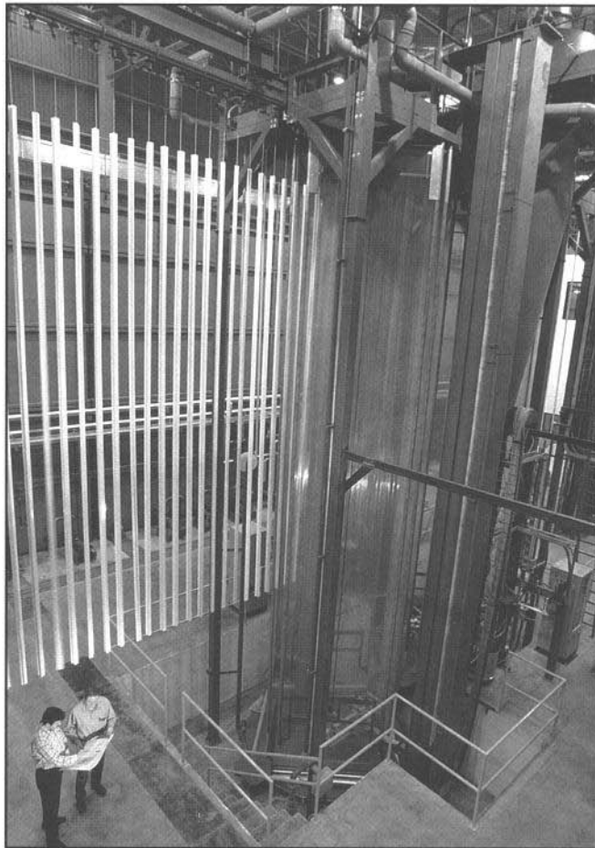
Figure 2. View of profiles entering first powder spray booth.
